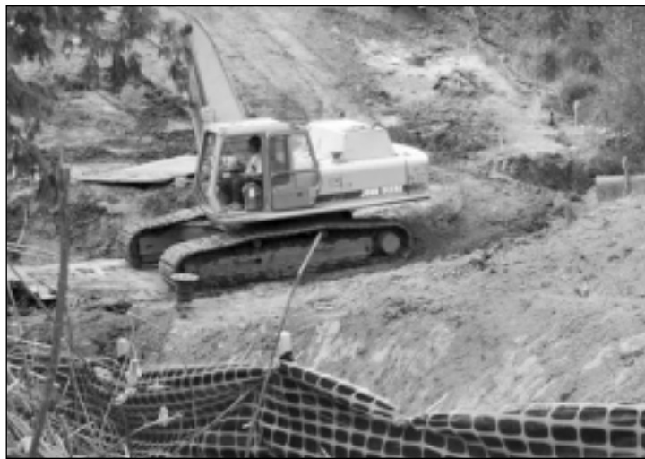
Construction of a road crossing over Summer Creek for the Murray Scholls Towncenter. Reacting to such developments has limited success. It is critical for citizens to participate in making the policy decisions that will ultimately determine where development can occur and whether natural resources are protected.
